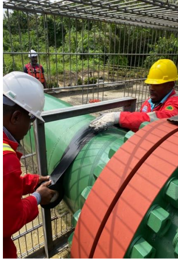
Sensor Installation on Field.
